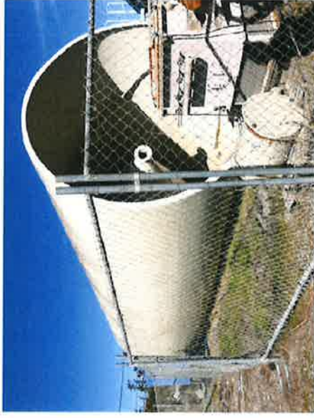
Lime Storage Silo
