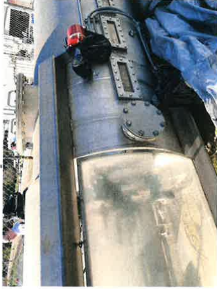
Pellet Reactor Column
